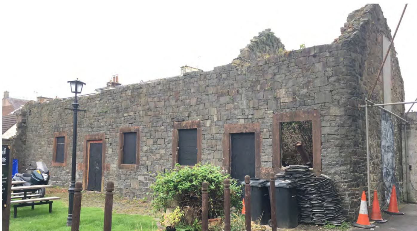
Derelict building on Rae Street, behind Buccleuch Hotel
